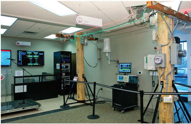
Utility Distribution Feeder, Substation and Control Center Components with Instrumentation
